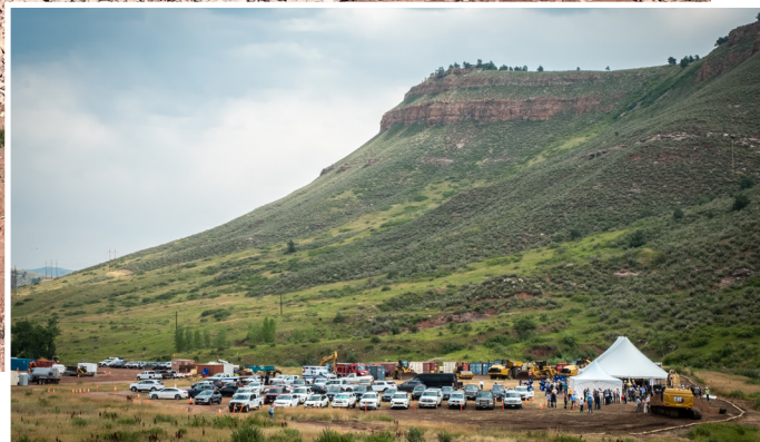
Rockfill placement on the main dam in August 2022. Inset: Groundbreaking ceremony in August 2021.
