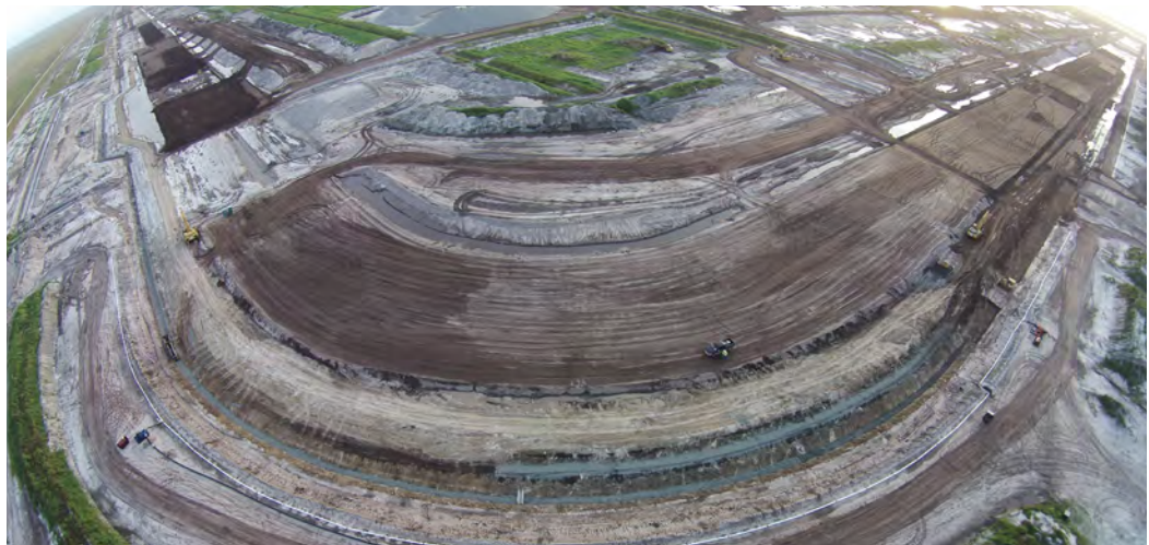
Crews complete the toe trench installation around the radius of the embankment.
