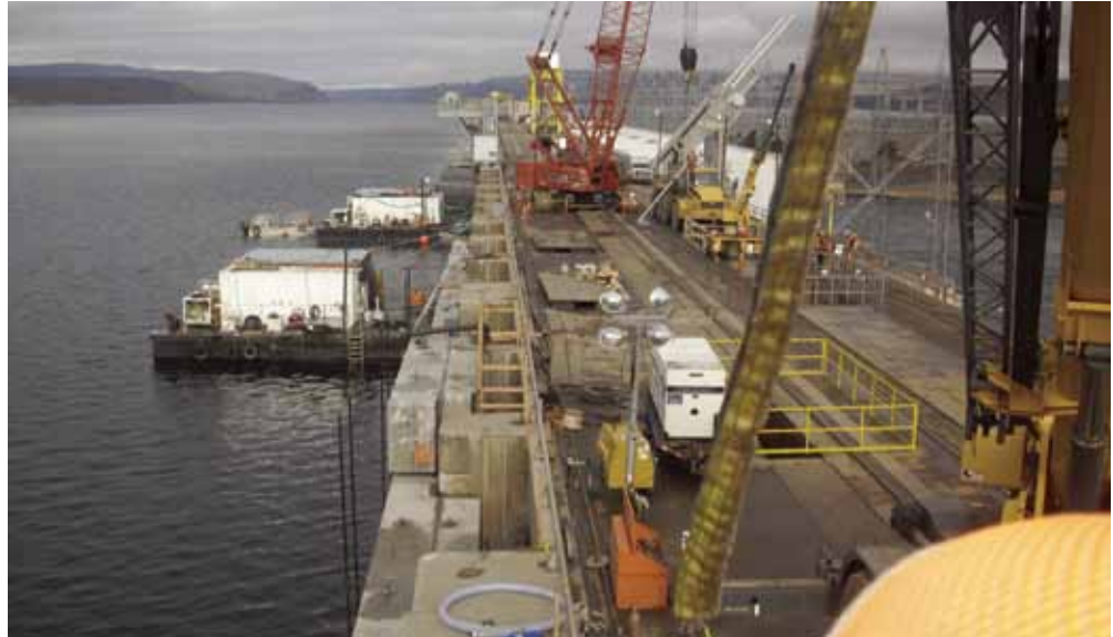
A view from the crane basket at Wanapum Dam shows dive barges with crews installing and bolting upstream stop logs on the left and downstream stop logs on the right.
