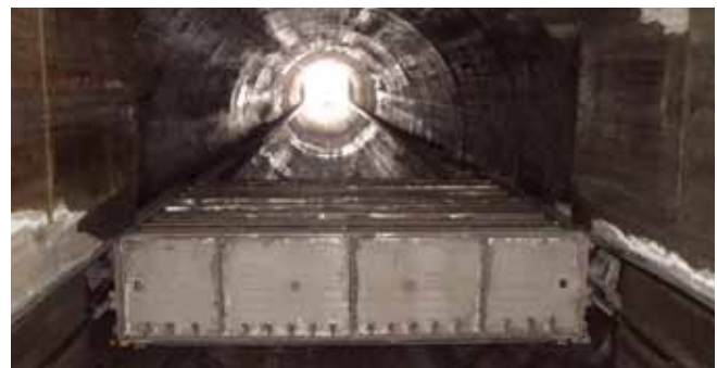
The isolation gate slides down the recently constructed shaft at the Lake Mead Project.
